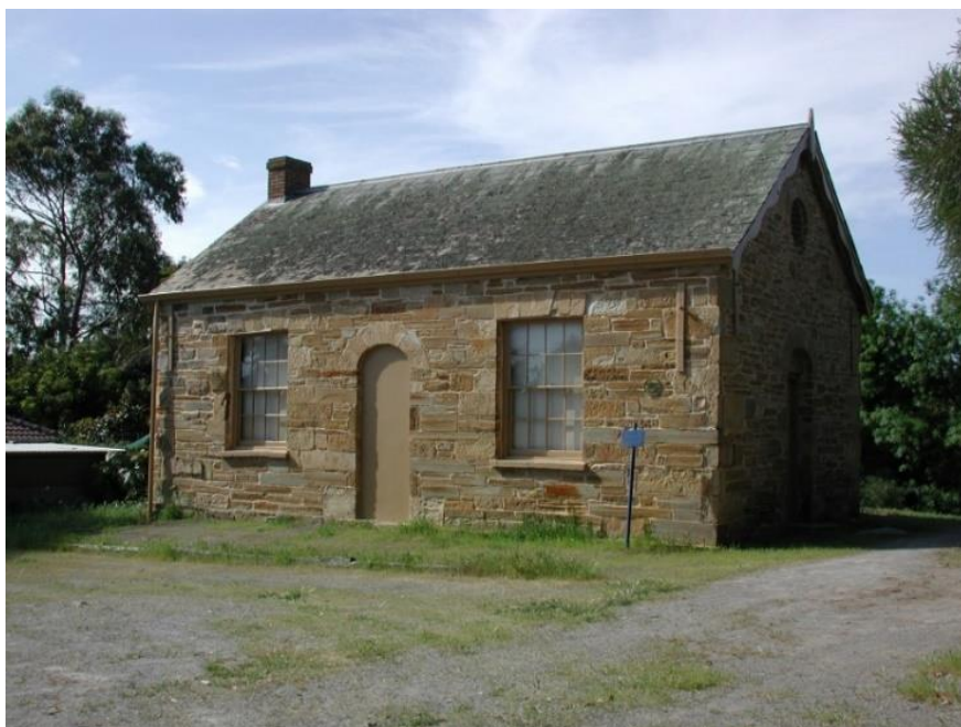
Former Council Chambers, also known as Former Bassett's Boys School (later Willunga Council Chambers) (SHP 10345), c.2000. Built 1862.
