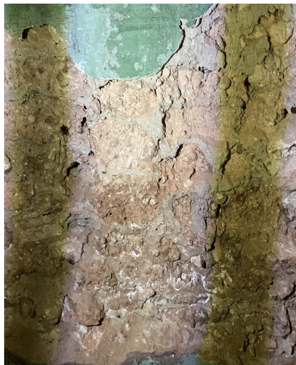
Degradation of the limestone on the inside of the northern wall.
