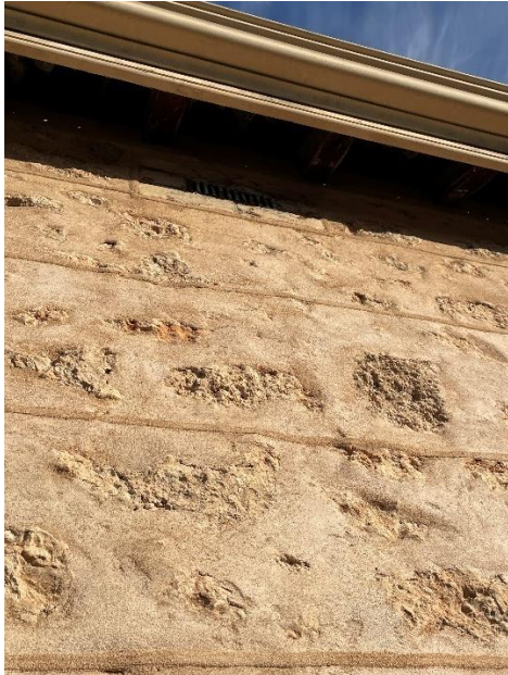
Close-up view of the repointing on the eastern wall showing that concrete has been used to render the limestone.
