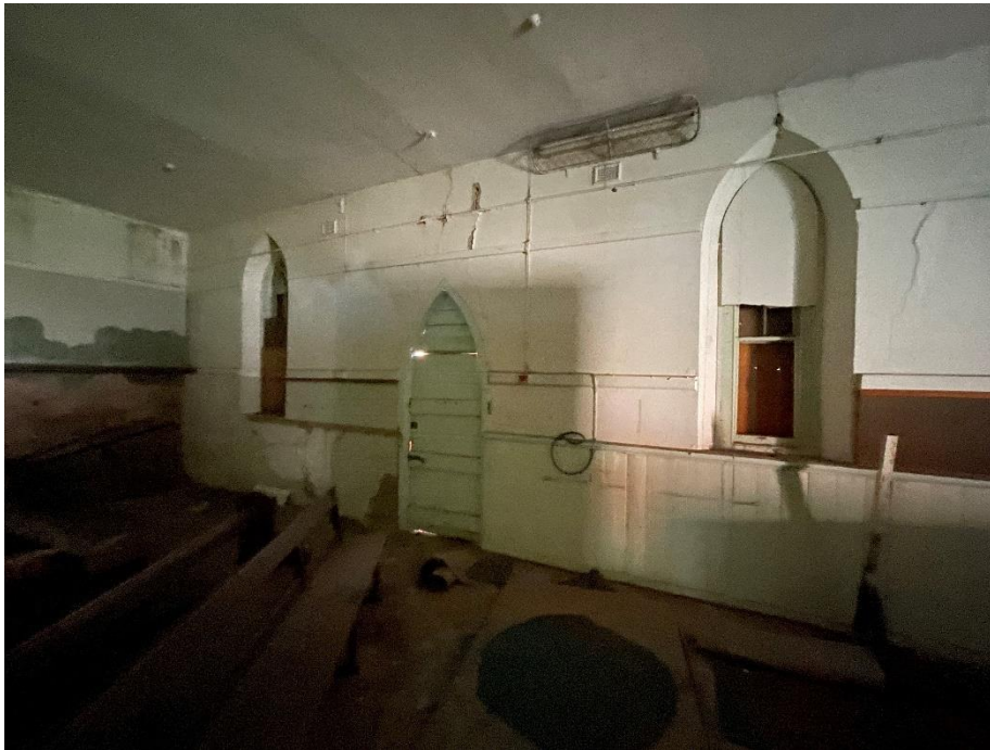
The interior side of the east-facing wall showing the original windows and entrance.
