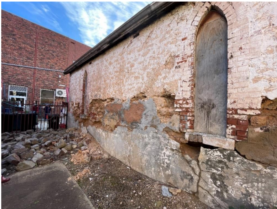
Part of the western wall showing considerable damage to the limestone walls, including a hole under the middle window.
