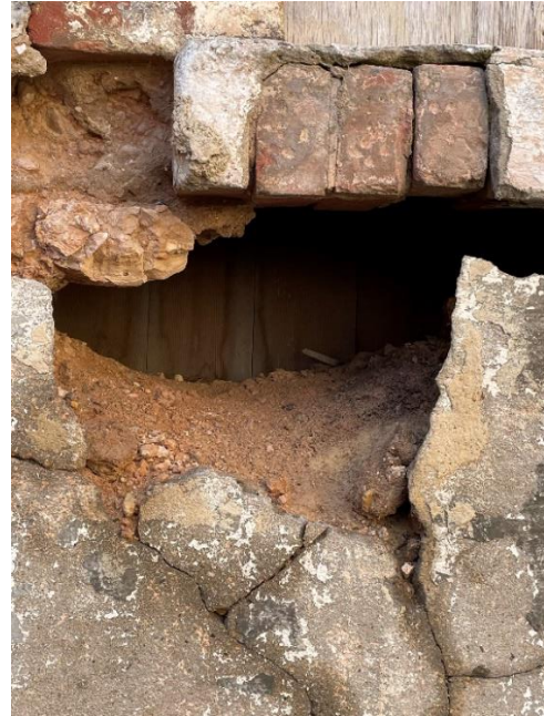
Close-up view of the hole underneath the middle window on the western wall.
