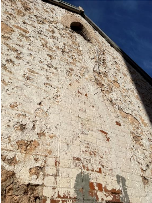
Northern wall showing a bricked-in window and louvred vent with pointed arch.
