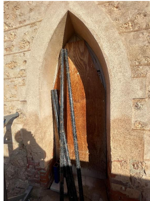
The original front-entrance on the eastern wall. The pointed-arch quoins have been rendered with concrete.
